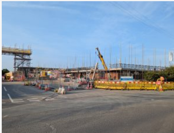
William Farr House – Redevelopment of brownfield site to provide extra-care affordable housing
